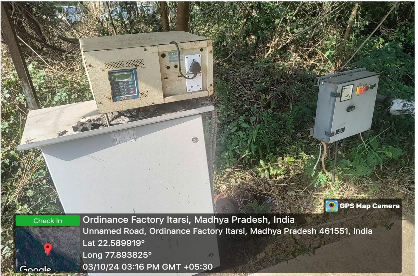
ETP Area of the plant
