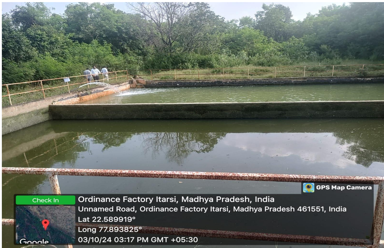
Treated water storage tank
