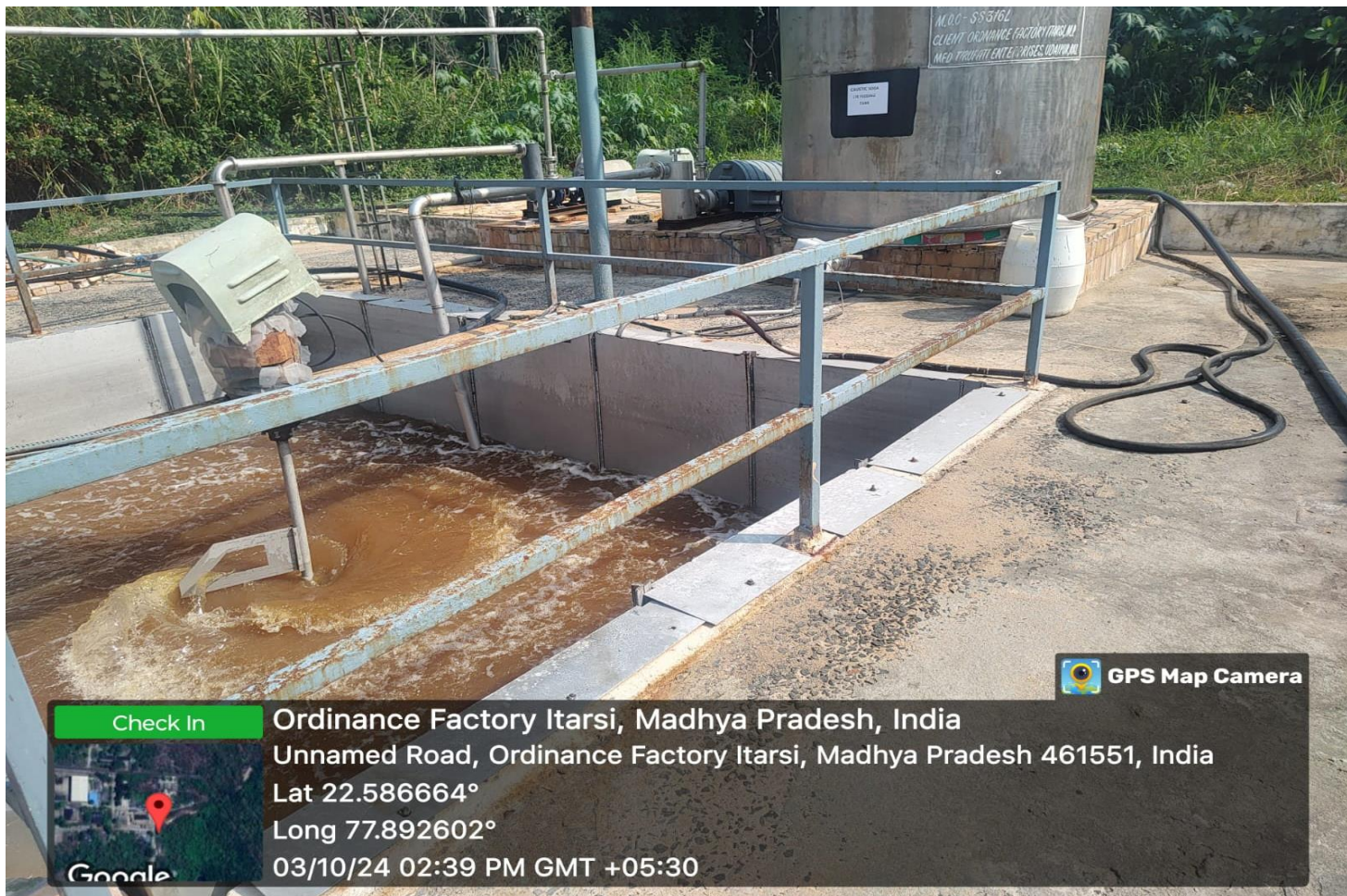
ETP Area of the plant
